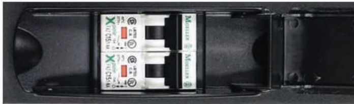
UL 489 hydraulic-magnetic circuit breaker on 30 Amp PDU.
